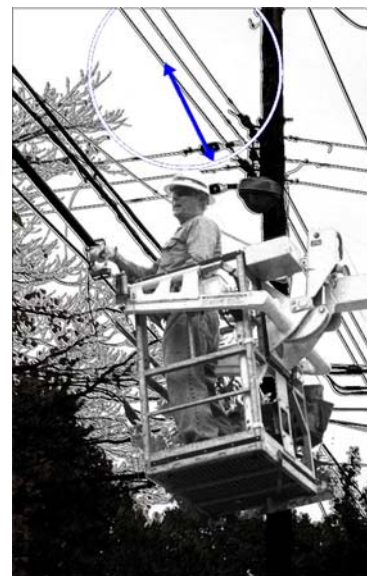
Min approach distance is 24" if this is a 13 kV power line.
